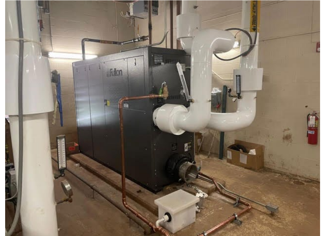
New Hydronic Boiler at CHS
